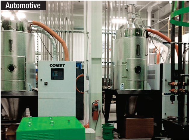
Two of four CDD-1200/700 dryers
