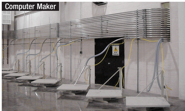
Low profile tilt tables and piping
