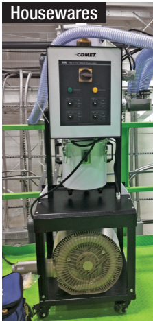
CAL 10HP vacuum system
