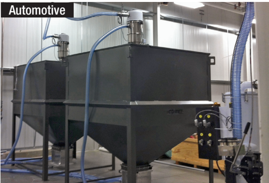
Two surge bins with two CHR receivers
